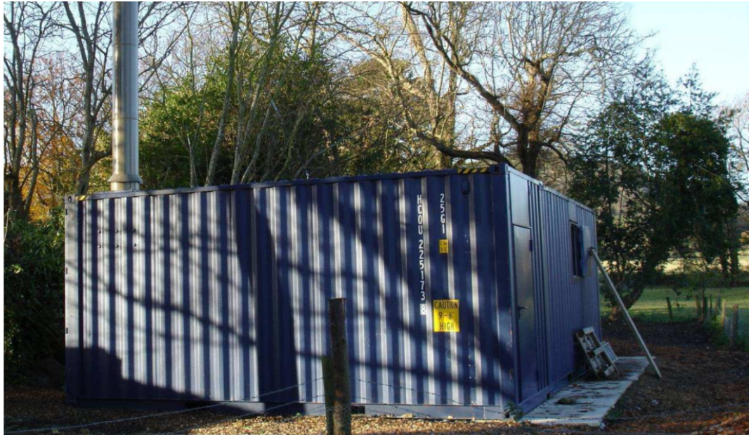
Figure 12 - Example installation - C/O Econergy
