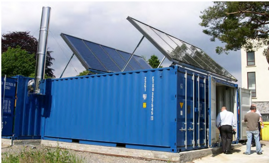
Figure 13 - Example installation - C/O Econergy
