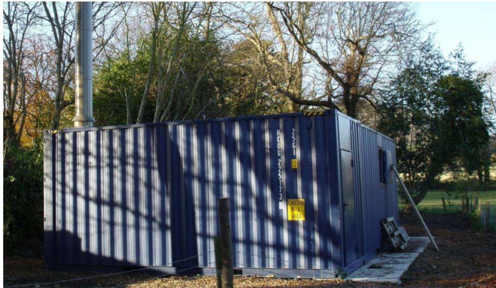
Figure 9 - Example installation of containerised biomass boiler (C/O Econergy)
