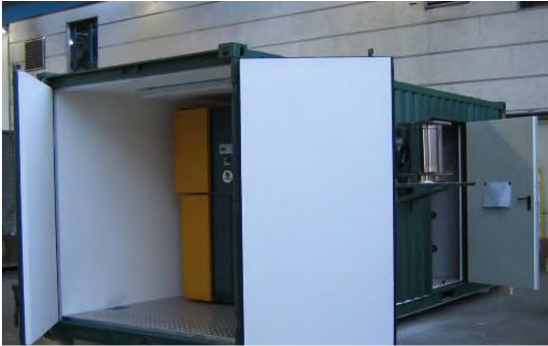
Figure 14 - Internal view of biomass boiler installation - C/O Econergy
